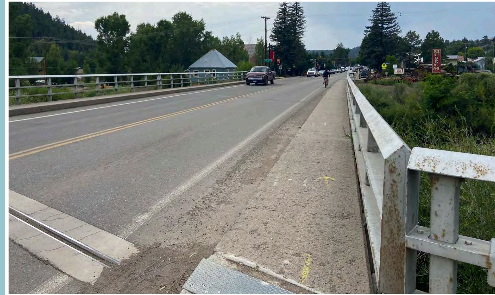
The Highway 160 bridge across the San Juan river presents challenges for people walking and biking.
